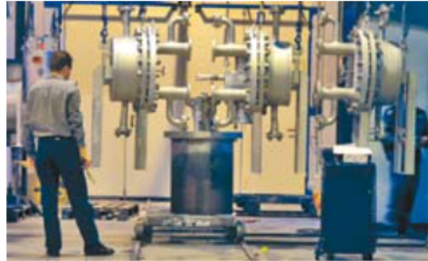
480 kW Raffinate Stripper Bottoms Cooler, PSHE 5HH-148/1/1
